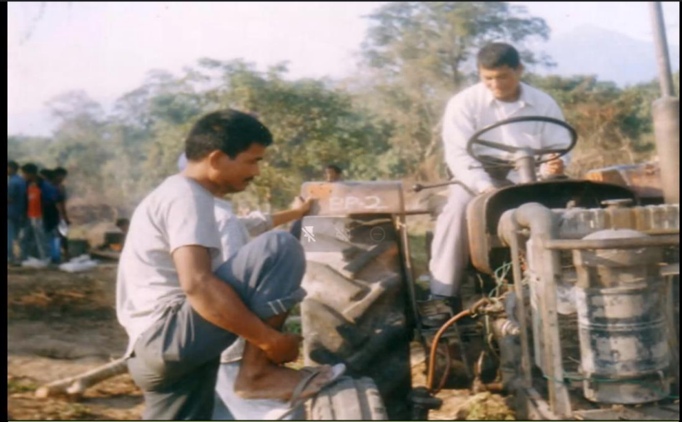
Ex-timber smugglers & Ex-BLT members on road construction work along with MMES volunteers, November, 2004
